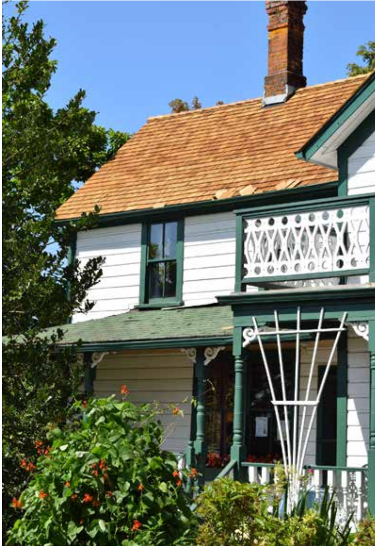
The Haney House roof is being restored to its original shingle finish.
